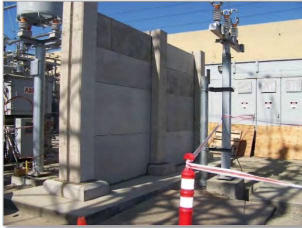
Physical Firewall at Electrical Substation
